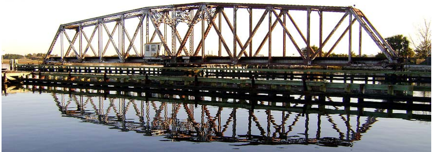
Swing span bridge over the Amelia River at Fernandina, Florida. Original Florida Railroad ROW, now First Coast RR. Bridge was barged from Palatka, Florida when FEC removed it and tracks over the St. Johns River.
